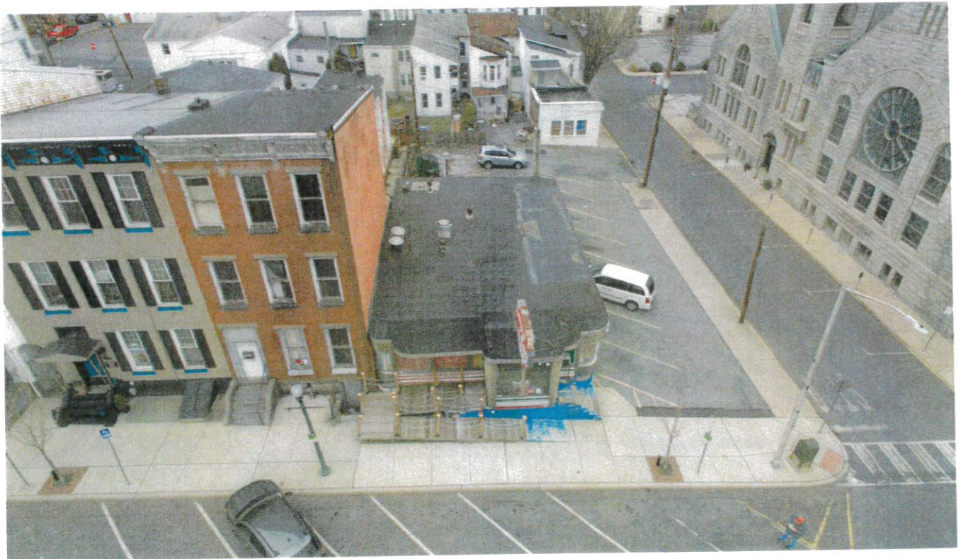
Aerial view of 402 W. West Market Street Diner showing the need for a complete roof repair since the underlayment is rotted.
