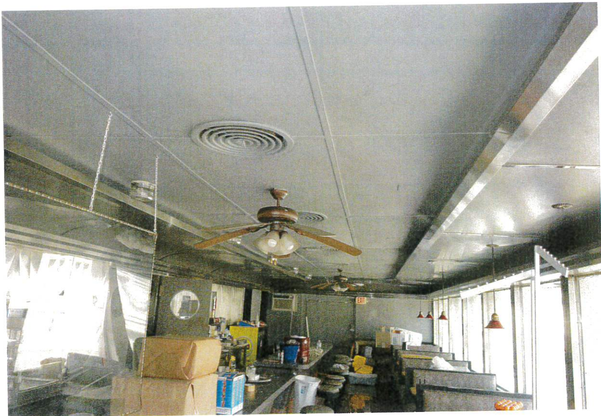
Showing the leaks in the ceiling
